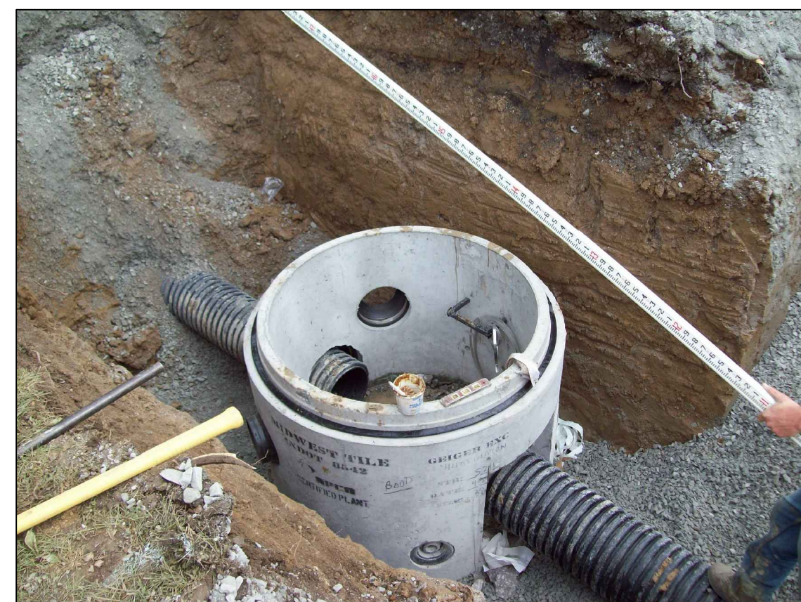
This is a storm sewer being installed. This type of material is HDPE Dual Wall pipe. It is normally installed for storm water applications. This particular picture is of a connection between two pipes via a manhole structure. Structures are placed at all bends or 400 foot intervals to allow maintenance crews an access to clean the pipes out when needed.
