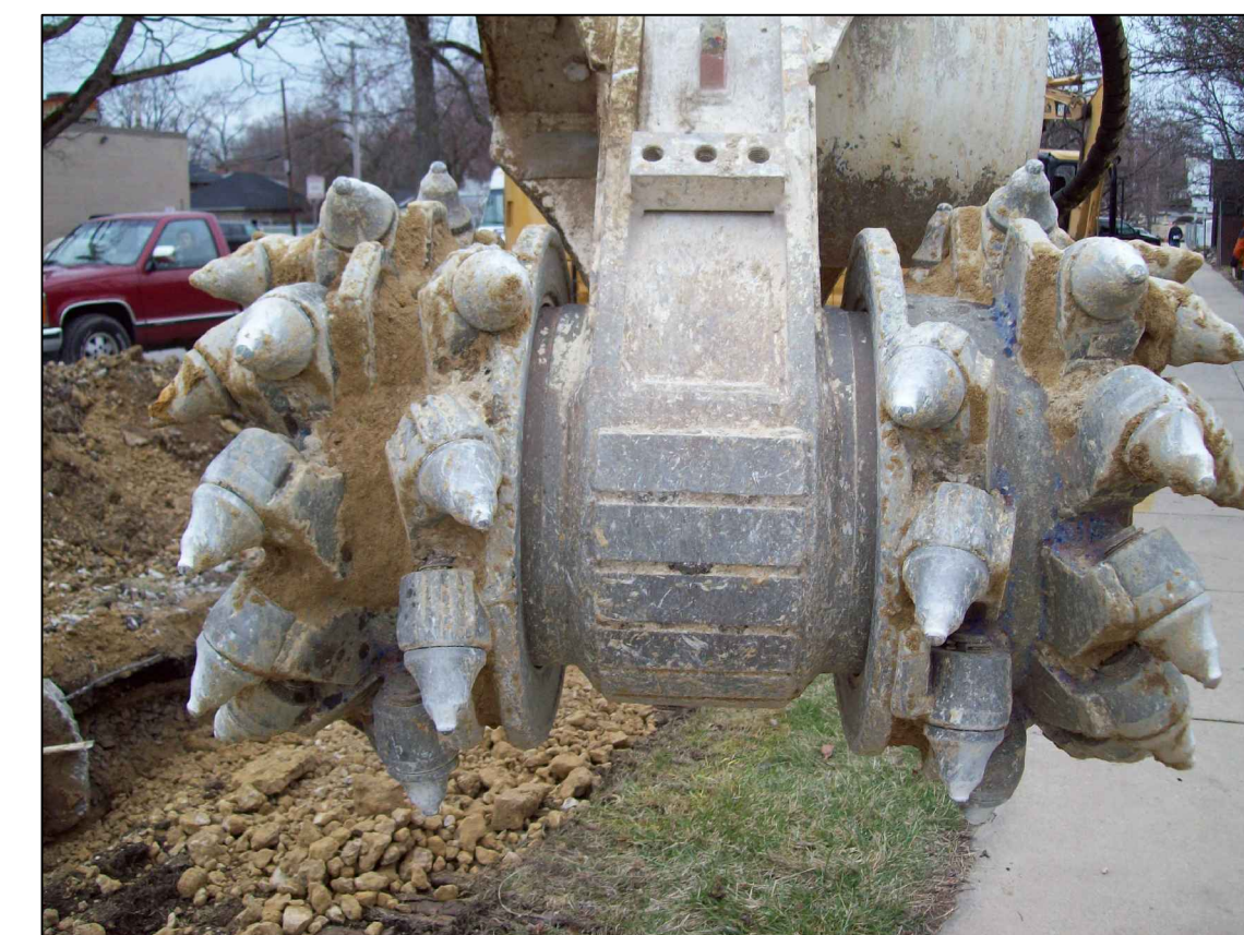
Throughout the job limestone was expected and encountered. There are many means of digging through limestone including blasting, hammering, grinding, and using rock teeth on an excavator. Depending on the hardness of the rock the grinder you see above was utilized within this job. To give an estimate it costs about $150 a cubic yard to grind out the rock.
