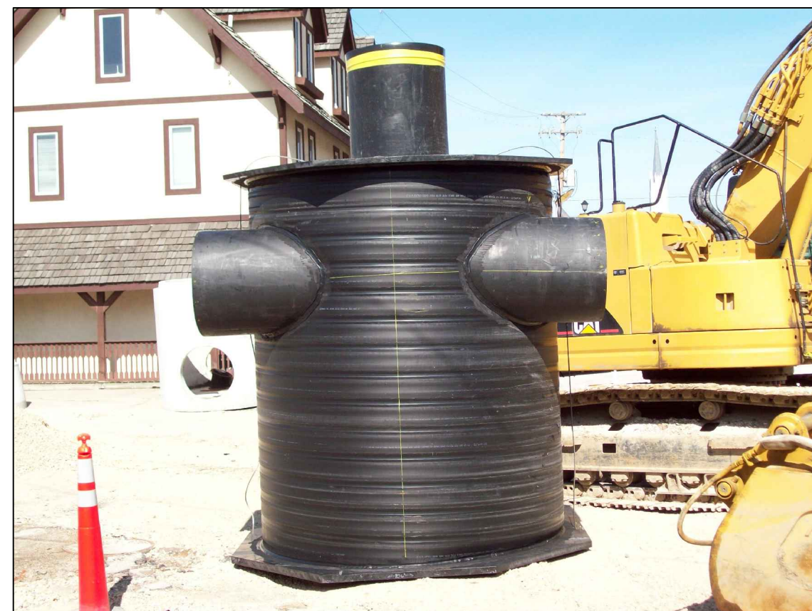
Hydrodynamic Separators were installed to clean the storm water as it passes through. Because of this the City was able to receive a lower interest rate on the loan due to the "green" that the separators incorporate.
