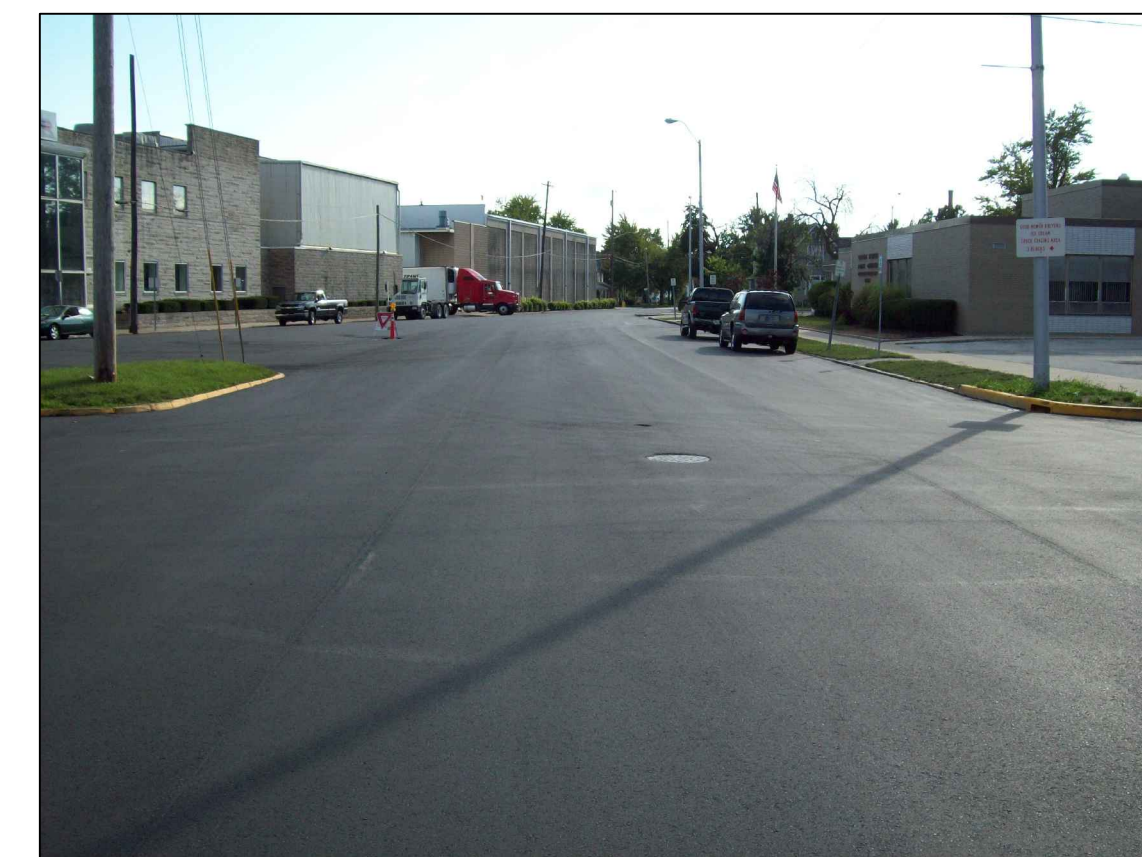
This is the finished product. All streets that are tore up within this separation project are intended to be repaved after the construction is done. The useful life of pavement is expected to be anywhere from 10 - 20 years depending on traffic. We expected some of these streets however have not been paved for well over 30 years.
