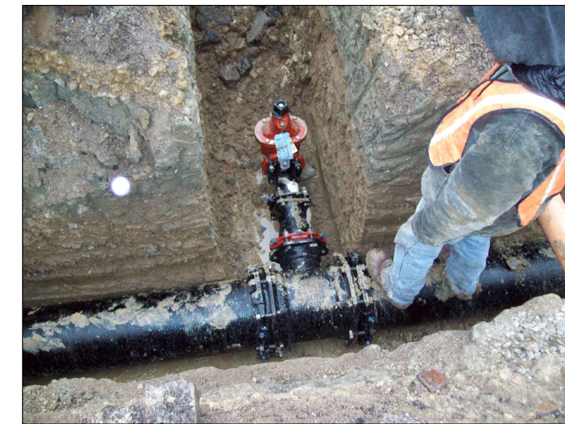
Due to water main conflicts, some water mains had to be rerouted. Per 10 State Standards all sewer mains must have a 10 foot horizontal separation from water mains. Other utilities were also encountered such as gas and electric lines. These conflicts were dealt with during the construction of the sewer.
