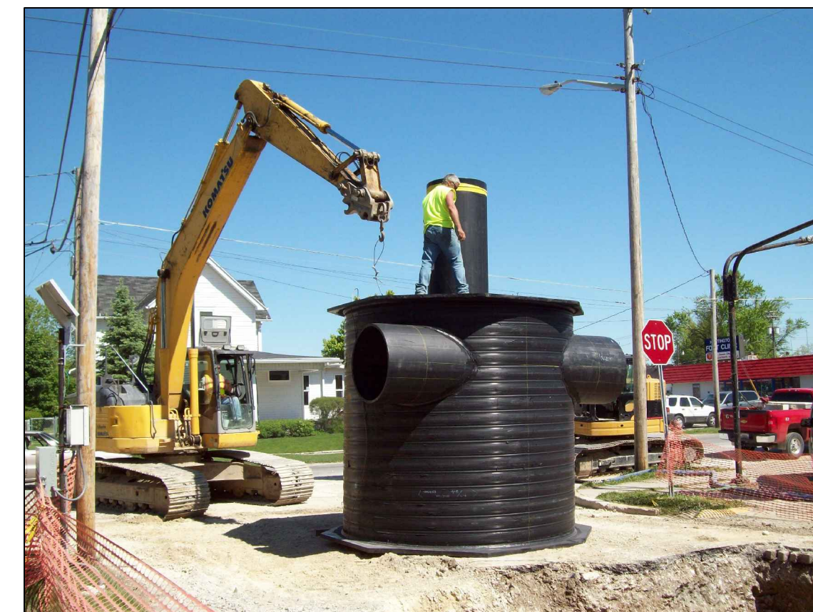
The Hydrodynamic separators were different sizes therefore larger pieces of equipment were utilized to install. This is a separator being prepped to be installed within the ground.
