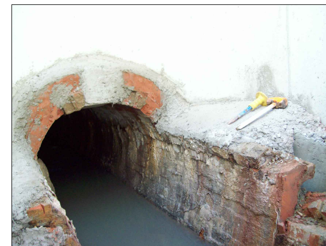
Brick sewers are extremely strong if all bricks remain intact, however if one brick is removed the integrity of the sewer comes into question so special care is used to ensure preservation of brick sewers that are not planned on being replaced.
