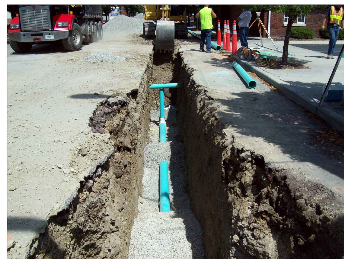
This is main line sewer being installed on Warren Street. Most phases the City installed new sanitary sewer, however in phase 1 the City installed new storm sewer. The decision for what type of pipe is installed depends on many factors including existing pipe size, depth, and condition.
