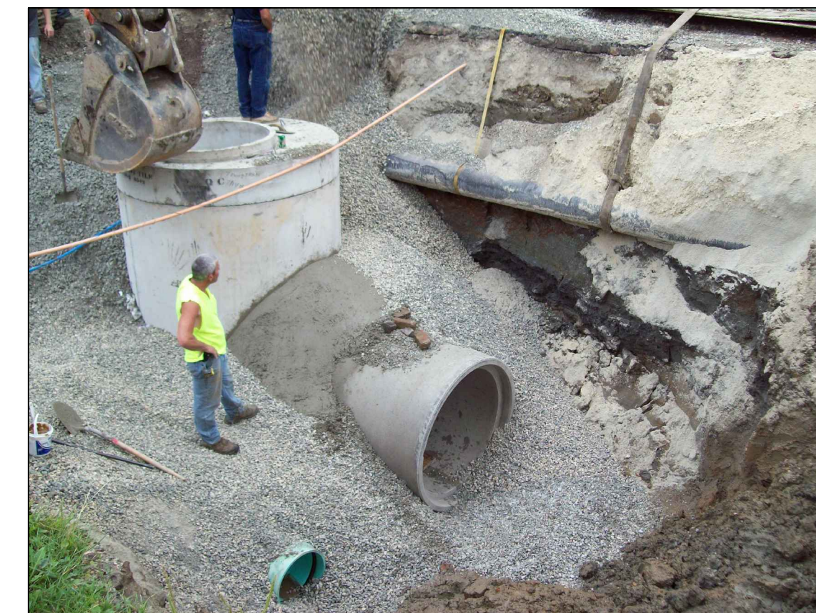
Many different types of pipe material is used depending on applications and locations. Here the center pipe is Reinforced Concrete Pipe. At the lower part of the picture you can see HDPE pipe in green. HDPE is an acronym for high-density polyethylene which is basically plastic.
