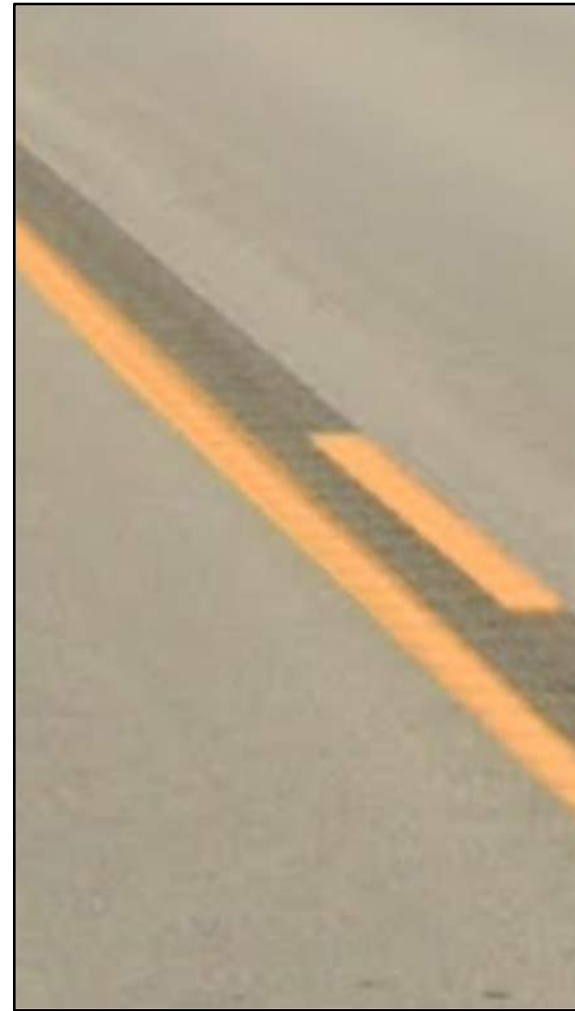
Sinusoidal centerline rumble stripes
