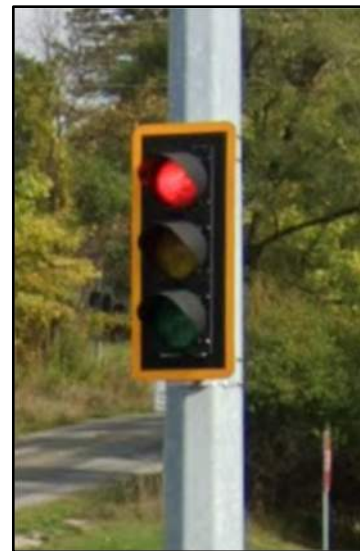
Pedestal mounted signal
