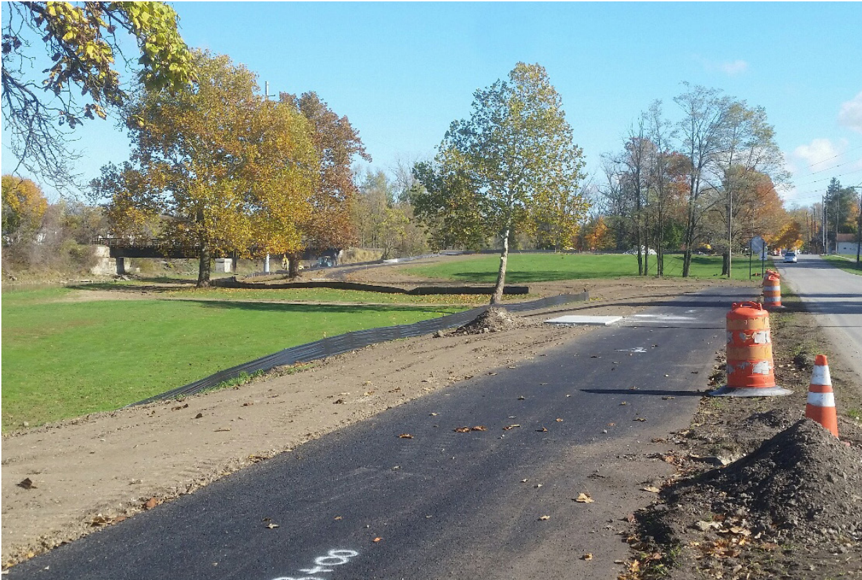
Figure 3-6: Development of a section of the Little River Trail in Huntington. Source: HCUED.
